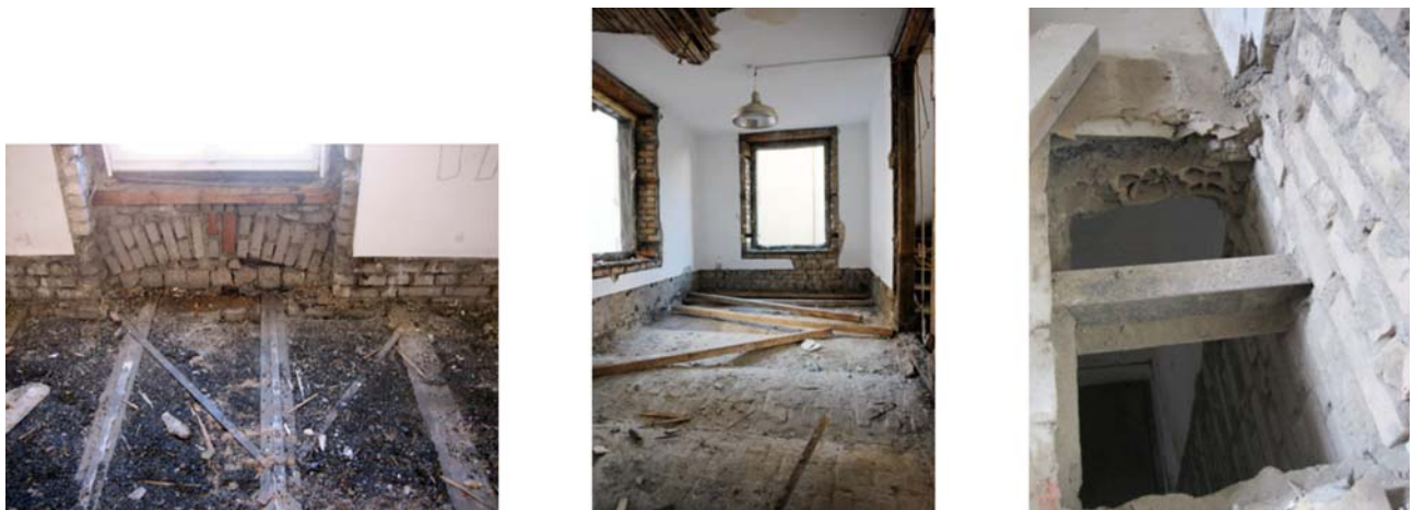
Figure 5: The construction of historical building is often complex and heterogeneous: Wooden beams running to a window alcove with a filled discharging brick arch. Grouted anchors of iron
