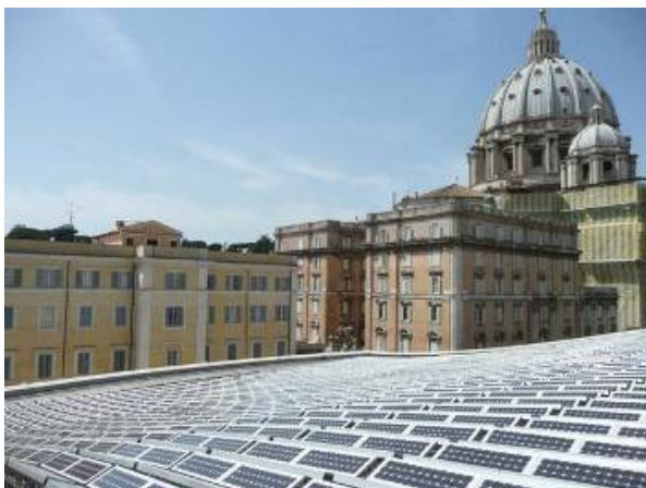
Figure 28: Large PV installation on the Nervi Audience Hall of Vatican City
