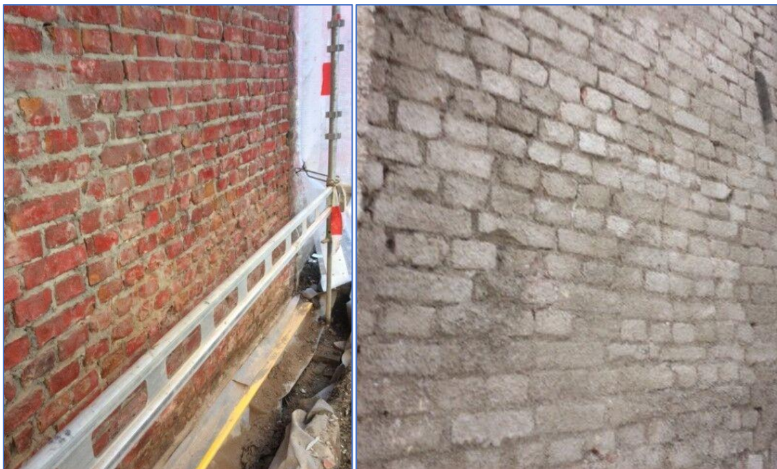
Figure 22- Image one: The clean surface, ready for application of the undercoat layer. Second image: The surface with an undercoat layer. When the undercoat is dry, a layer of Fixit222 can be applied (Source: Boligbygg).
